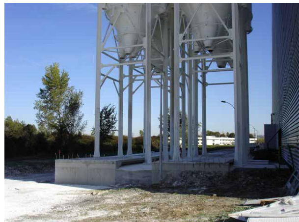
Mounting under silos
