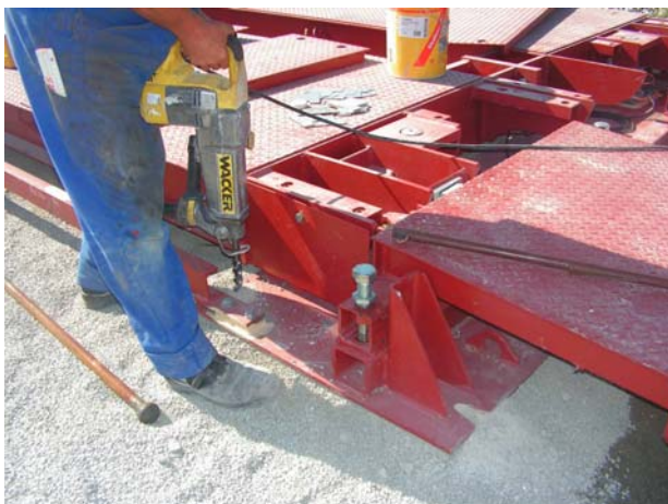
Step 6: Drilling and hammering in of the floor spikes with the heavy duty hammer drill for foundation securing
